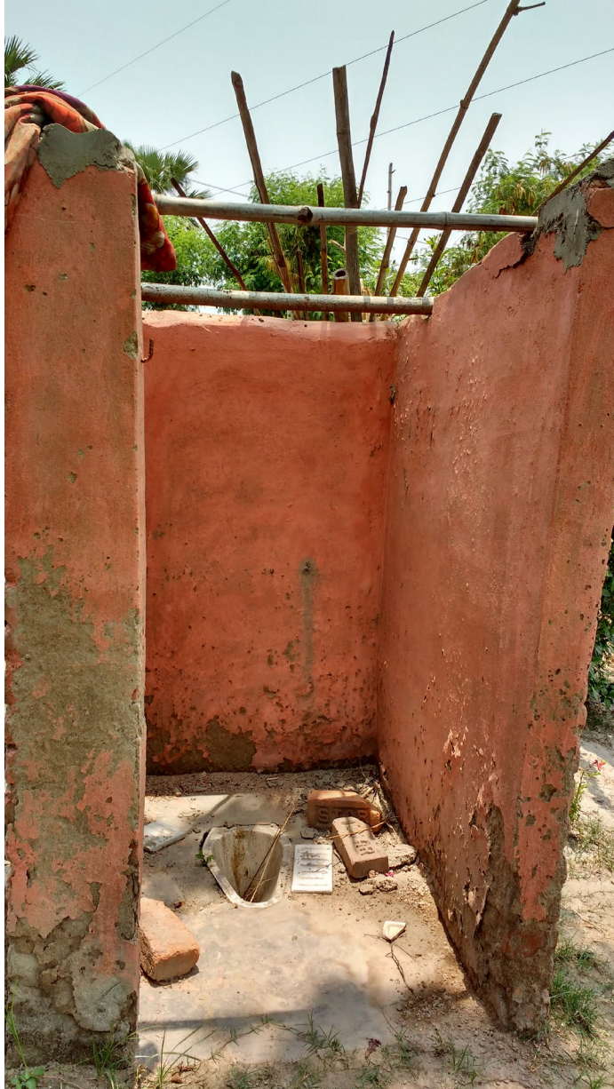
Figure 6: Contractor built defunct latrine, Gopalganj
