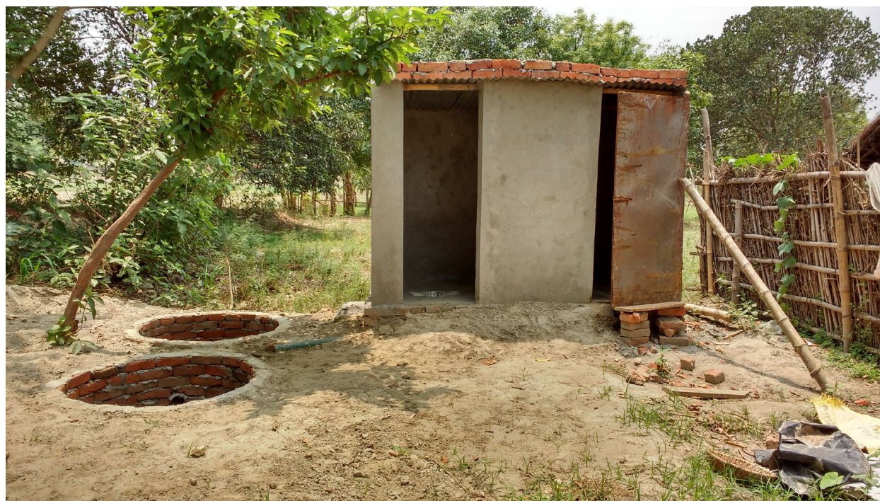
Figure 7: Contractor-built, incomplete latrine, Paschim Champaran
